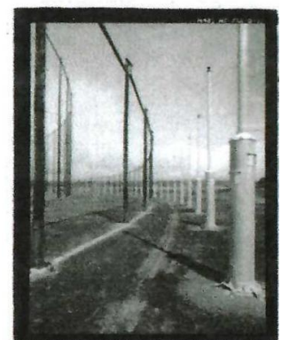
25 ft high-band reflector screens on the left. behind the high-band monopole antenna at right.
