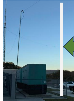
(R) This photo shows the new location of the HF tower supporting the OCF HF antenna.
