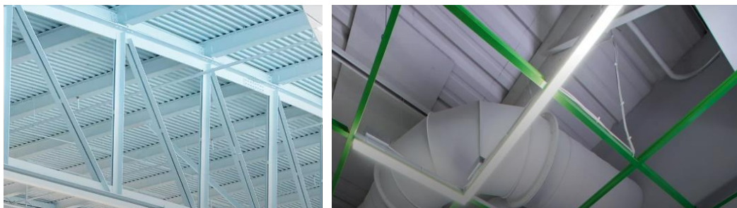
The photographs above show typical commercial construction techniques used at most MCPS school Shelters. This type of roofing structure significantly attenuates MERT radio transmissions when the antenna is located inside the building. For best results, move your radio and emergency antenna to areas with large windows or glass type doors.
