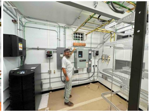
Interior photo of new communications bldg. showing state-of-the-art facilities with the interior lightning protection grid and high-capacity UPS.
