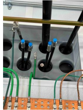
Photo of new antenna cable entry plate showing all four MERT cables. (Notice the huge grounding plate.)
