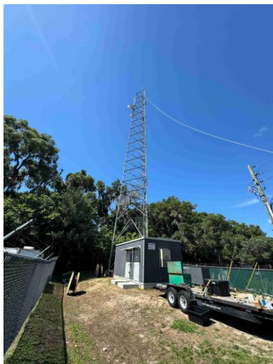
Tower has had all old cables and antennas removed. Now ready for all new equipment.
