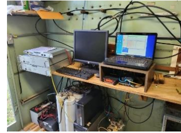
MERT Repeaters at Sheriff Office communications hut
